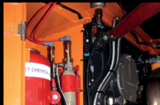
Fire suppression system
