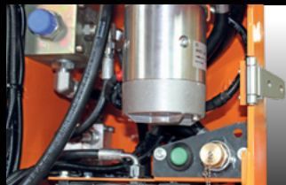
Oil fill pump
